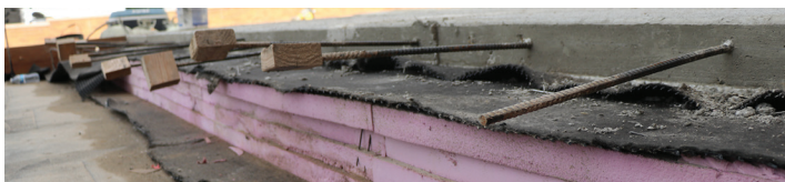
PRMA split slab assembly showing reinforced concrete topping slab over XPS with drainage board installed above XPS to promote vapor diffusion.
